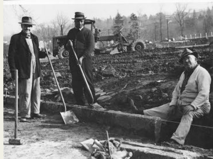
Photo of workers on the construction of the Tappan Zee bridge from Westchester archives.
