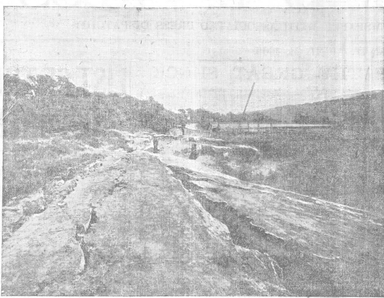
SCENE NEAR SALINAS, SHOWING BREAKS AND FISSURES IN ROADWAY. ONE BREAK IS HIGHER THAN A MAN'S HEAD.
