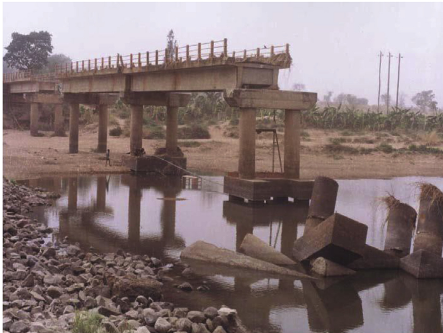
Fig. 2. A bridge damaged by floods in the Upper Niger River basin. Photo by: Andre Kamga Foamouhoue.
