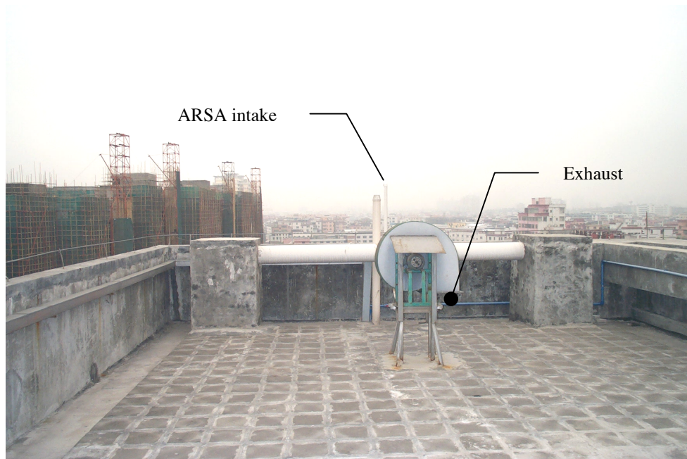
Figure 2. ARSA intake and fume hood vent location
