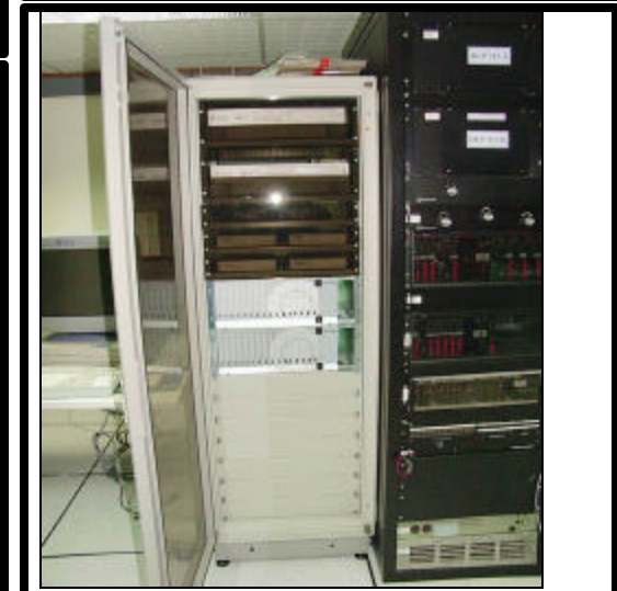
Figure 11. Front of new equipment rack at CRF, primary and back-up DAC on top, two each authenticators below DAC, 4 each RM-4s below authenticators, CRF communications modems below RM-4s. Older AFTAC rack to the right.
